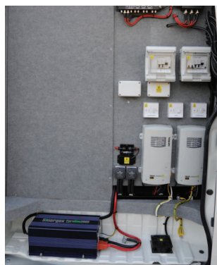
Easy Access to Power System
